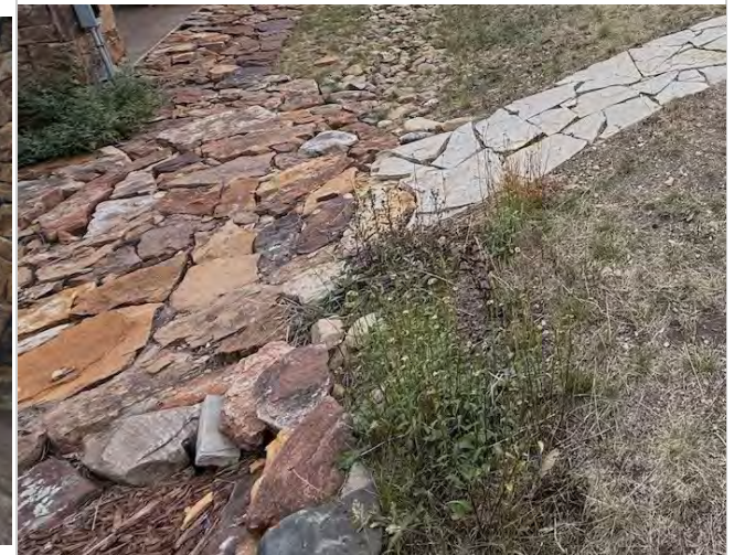
Photo 6: Patio, walkway and firepit very uneven and unsafe
