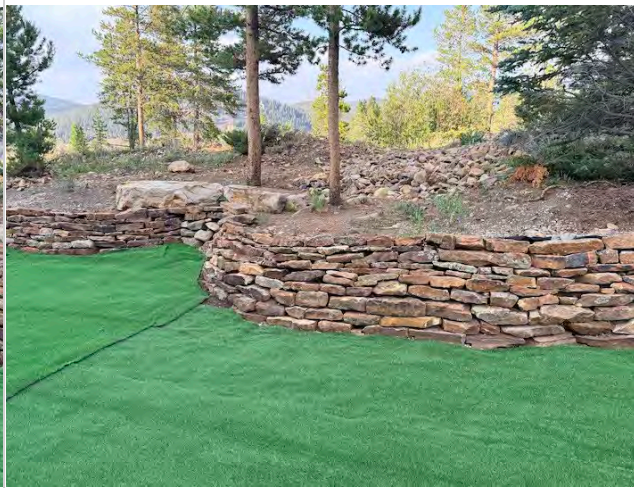
Photo 8: Retaining wall portion near previously existing fire pit. Rocks are assumed to be in the same location which show the amount of grade disruption.
