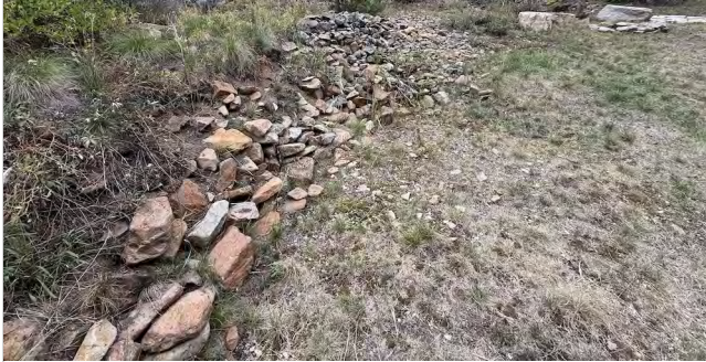
Photo 1: Collapsed Retaining Wall
