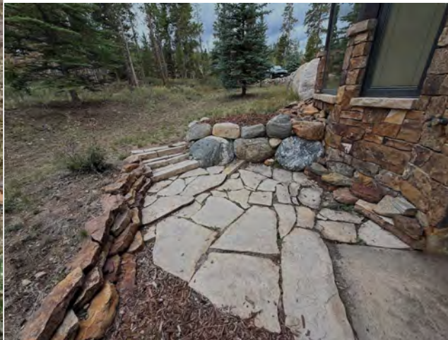
Photo 5: Patio, steps and retaining wall very uneven and unsafe
