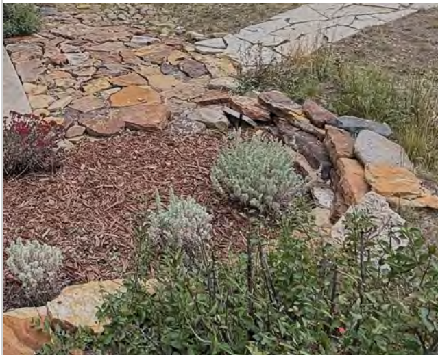
Photo 4: Patio, retaining wall and walkway very uneven and unsafe
